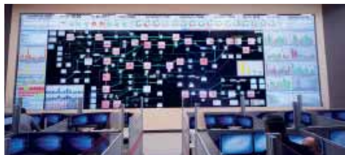
Russian Railways operator JSCo has installed a large-scale video wall in its Moscow transport hub centre. Integrator AMS selected a 11x6 video wall with Peerless-AV's DS-VW765-LQR mounts to enable the control centre to visualise critical transport network data in realtime from its workstations.
